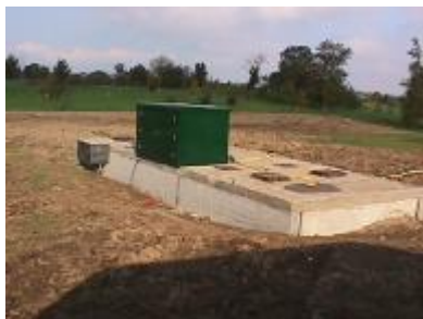
Aeration Tank at St. Margarets Golf Course, St Margarets, Co. Dublin
