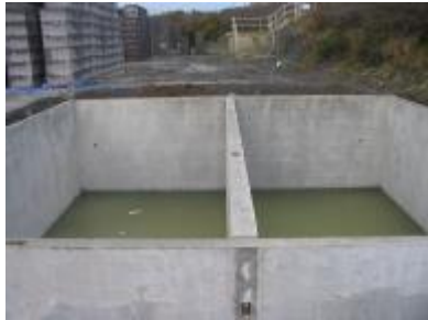
Water Tank at Taghart, Co. Cavan
