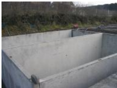
Attenuation Tank at Ramsfort Park, Gorey, Co. Wexford
