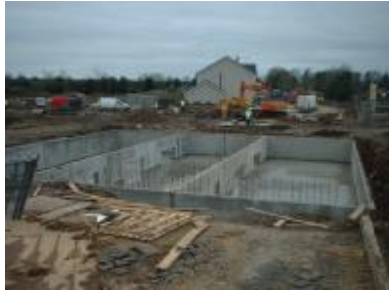
Attenuation Tank at Walshtown, Co. Kildare
