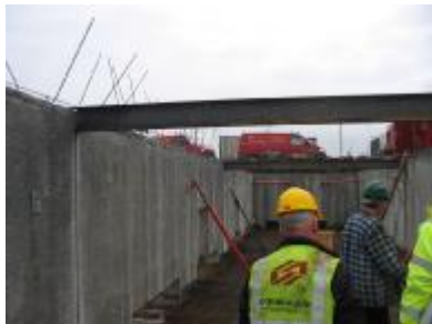
Attenuation Tank at Cornacassa, Co. Monaghan
