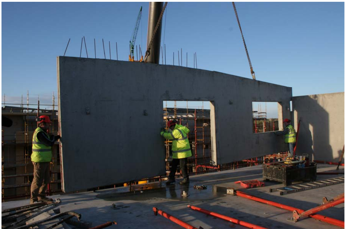
Walls dropped into position – T25 Bars line up with tubes in wall
